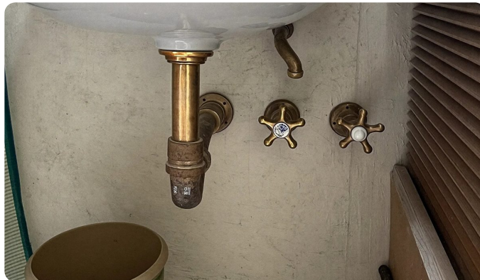
2. Corroded pipework and ageing isolation valve under the basin
