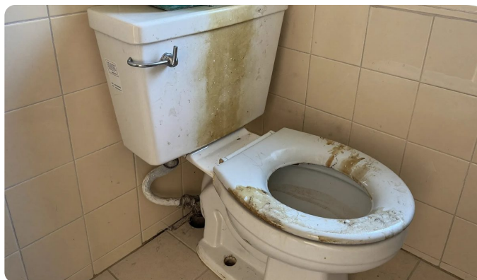
4. Existing toilet stained, cistern connection ageing
