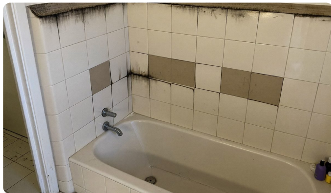
2. Grout blackened with mould along the top course
