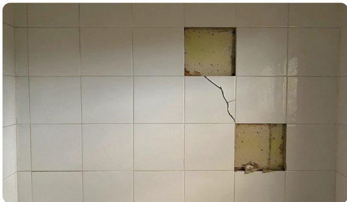
1. Cracked and missing wall tiles above the bath, adhesive exposed
