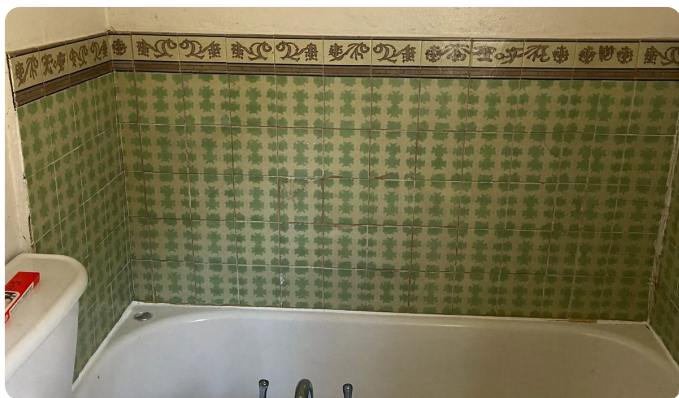
3. Existing tiling dated and discoloured throughout
